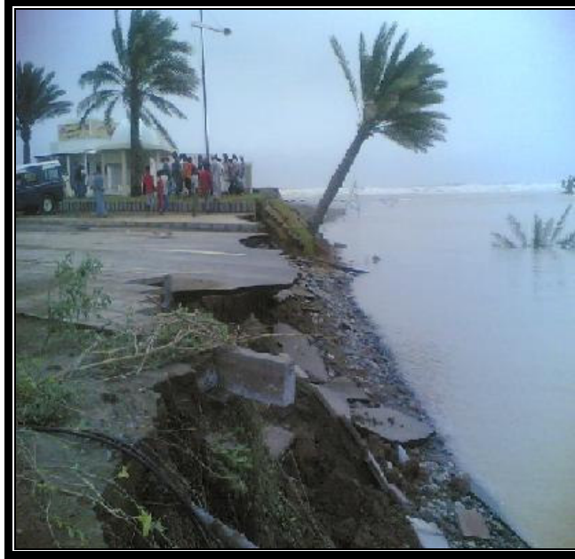
Photo (2) damages on Alqurm beach
