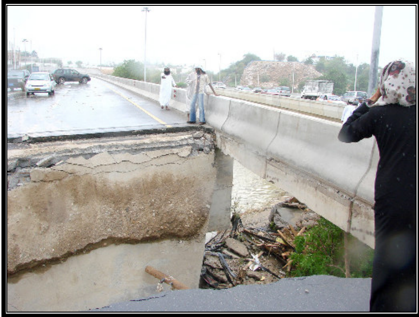
Photo 1: the damaged part of the bridge
